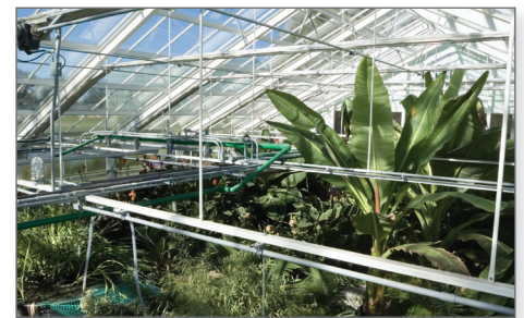
Tropical plants growing inside the greenhouse of the Solar Aquatics Wastewater Treatment have a key role in the water treatment process.
